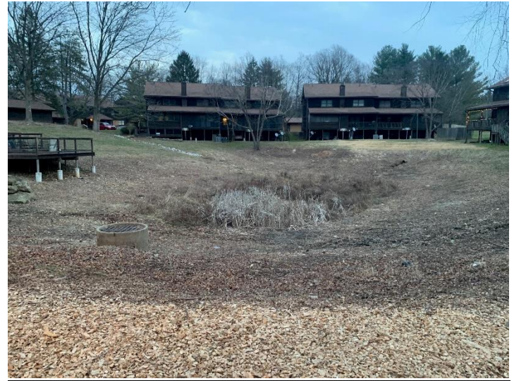
The common pond area that needs to be repaired
