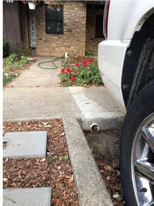
A drain that was repaired similar to the proposed community wide drainage project for 2023/2024
